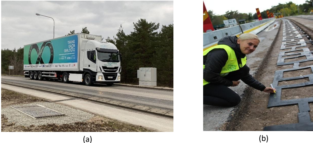
Figure 7 Dynamic Wireless Charging for an Electric Truck (a) dynamic wireless charging lane in Gotland, Sweden for long haul truck (b) transmitter coil in the dynamic charging lane before asphalt.
